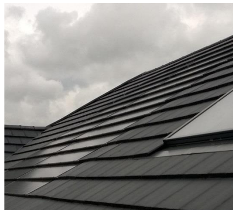
↑ Above: Solar PV panels generating around 640 kWh per year
