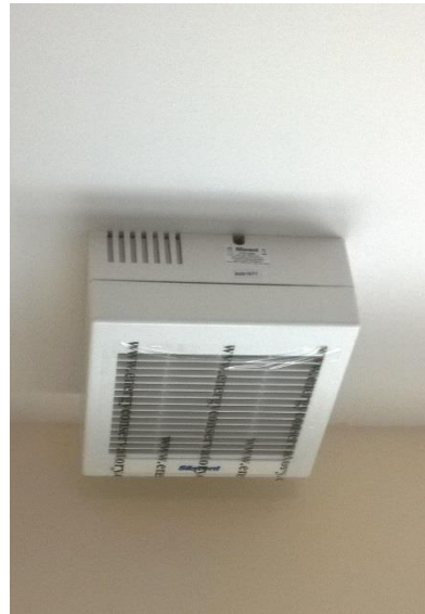
↑ Above: Silavent standard centrifugal fan in Kitchen
