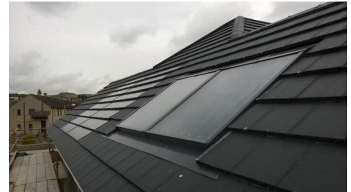
↑ Above: Solar water panels – 2 panels to service your flat
