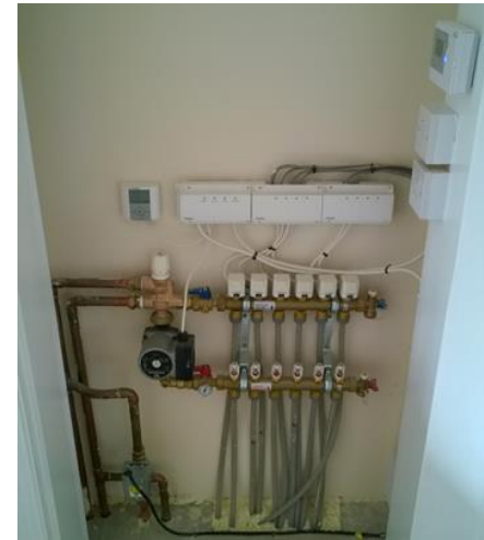
↑ Above: Manifold underfloor heating controls
