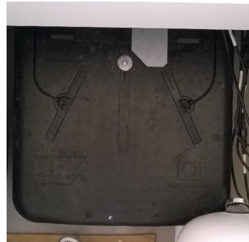
↑ Above: Silavent Polypipe HRX MVHR unit.
