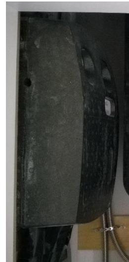
↑ Above: Solar panel pumps – do not adjust
