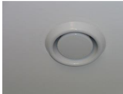
↑ Above: Polypipe extract and supply vents
