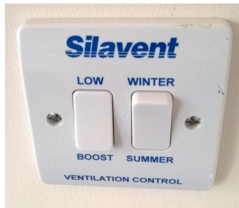
↓ Below: Silavent ventilation controls
