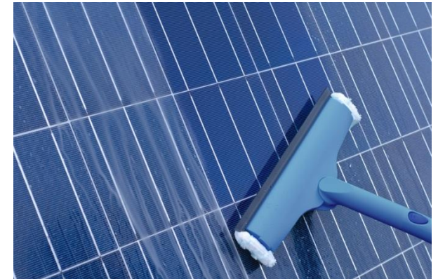
↑ Above: Solar PV panels require washing once a year to maintain efficiency
