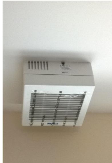
↑ Above: Silavent standard centrifugal fan in Kitchen
