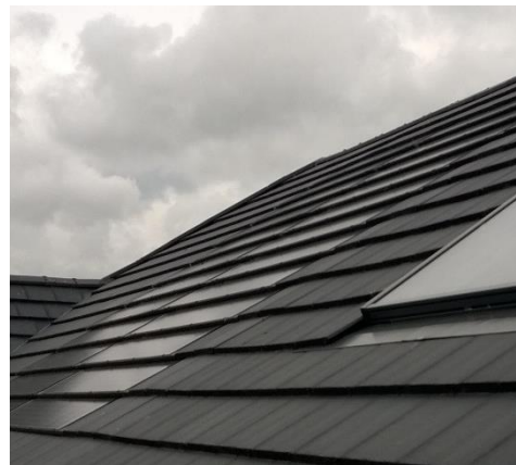
↑ Above: Solar PV panels generating around 950 kWh per year
