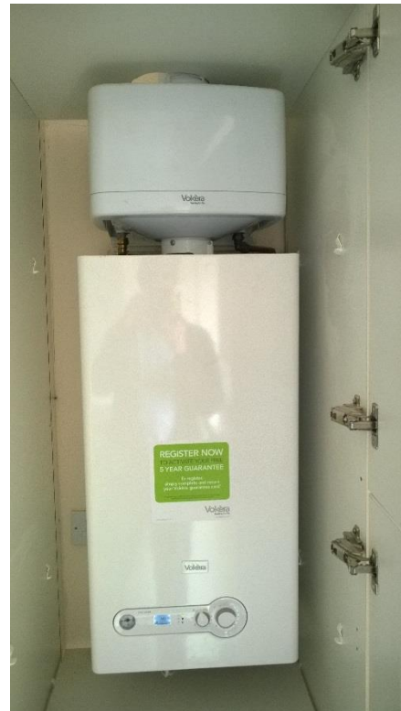
↑ Above: Vokera Unica i28 with a Flue gas heat recovery unit.
