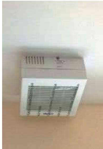
↑ Above: Silavent standard centrifugal fan in Kitchen
