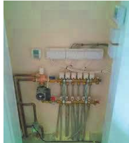
↑ Above: Manifold underfloor heating controls
